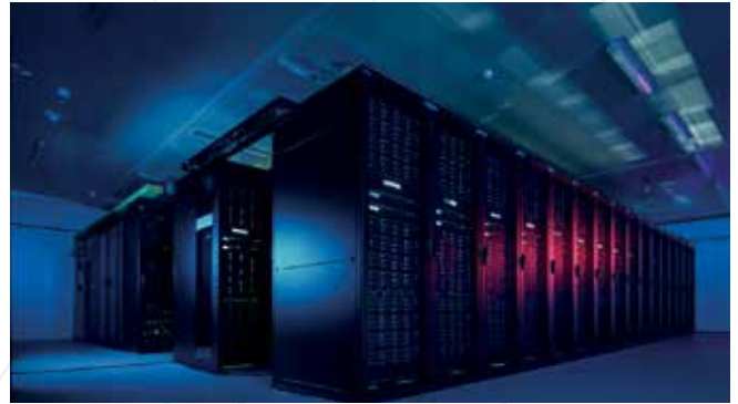
Figure 4. Data Centre Excellence
