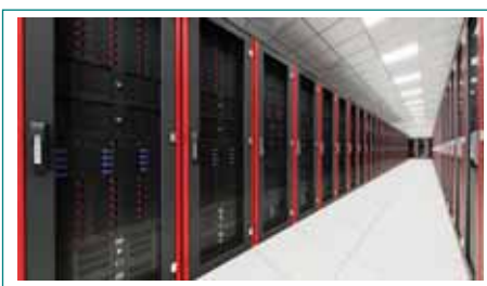
Figure 1. Exyte Data Centre Project
