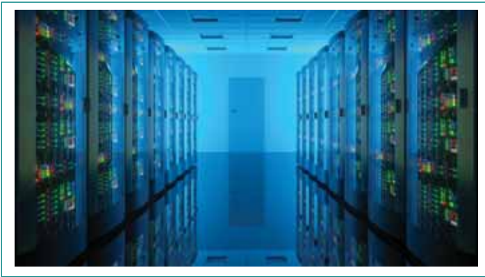
Figure 2. Exyte Data Centre Server Bank
